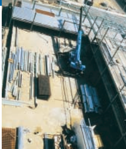
While one half of the carpark was being built, the other half was used for storage of materials.
