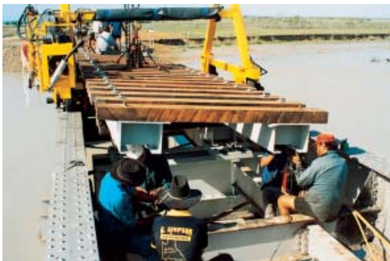
Figures 12 and 13. Erection of new spans from travelling gantry at St Lawrence Creek bridge.
